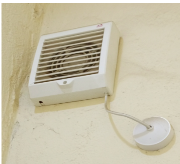
Figure 2. Wall-mounted ventilation system.
