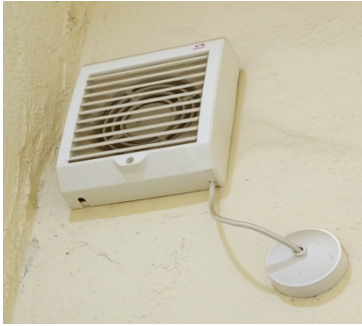
Figure 2. Wall-mounted ventilation system.
